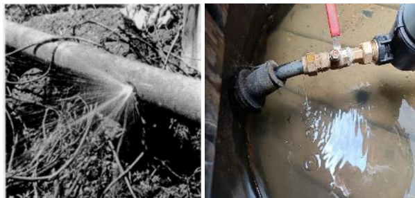
Figure 2.2. Leakages on a supply main (street main) and a house connection pipe (Losses in Water Distribution Networks – A Practitioner’s Guide to Assessment, Monitoring and Control, Malcolm Farley and Stuart Trow, IWA Publishing, 2003)
